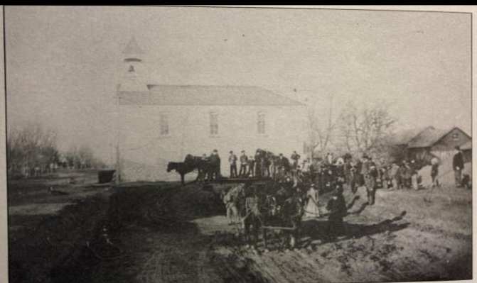
Excavation begins for Woodman Hall, located south of Old City Hall where it served as a community center until its removal in 1978.
